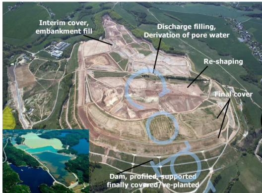
Fig.5 “Trünzig”-site, different parts of cover design, small photo: water covered tailings pond, Rio Algom/Quirke site/Elliot Lake/ Ontario/ Canada; source: BHP Billiton, 1999 and M. Lersow/Wismut GmbH May 2007
